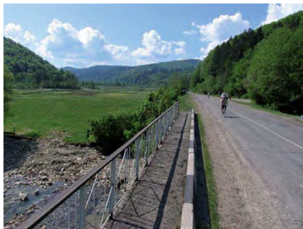
Figure 44. Bridges may become obstacles for wildlife, but conversely, they can be adapted to facilitate the passage of wildlife under roads.
