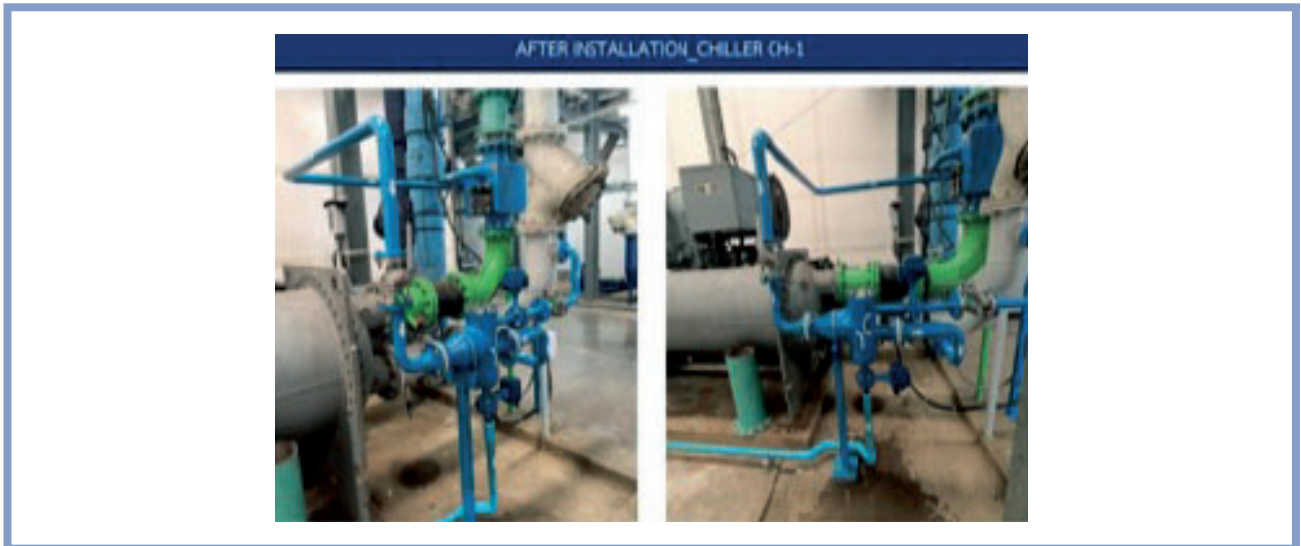
Remarks: Refrigeration system (Chiller)
